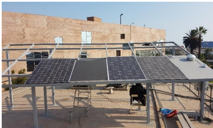
Fig. 1: Outdoor station for characterization of PV modules and the environmental sensors.
