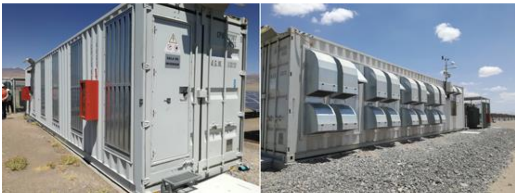
Fig. 1: FIMER MS3000 Inverters room, inside it contains four FIMER R7500TL inverters.
