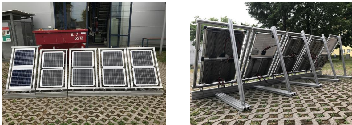
Figure 2: Pre-commissioned PV system cooled with PCM Absorbers in Dresden, Germany
