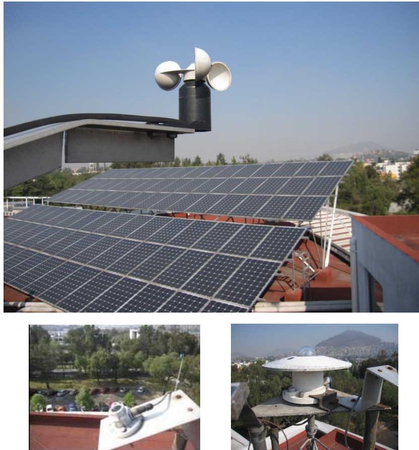
Fig. 1. The upper figure shows a section of PV module array and the anemometer installed in CINVESTAV, Mexico City. The lower pictures shows; the thermopile-pyranometer MS-602 arranged at POA (left) and right, the horizontal pyranometer.
