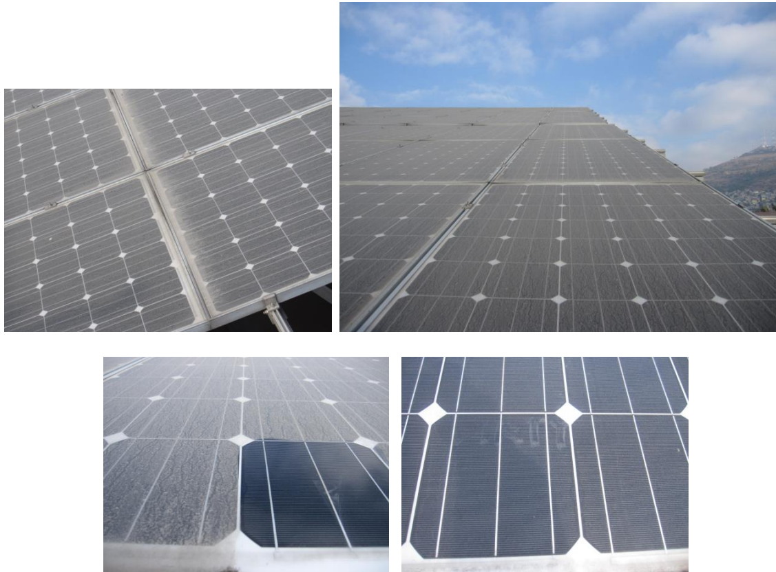
Fig. 4. Aspects of dust accumulation on the PV array; before (lower-left) and after (lower-right) rain fall. Both, the upper image shows the part of soiled PV-module array which is fixed at the angle of 20° from the horizontal-plane. In a lower-left also shows the soiled module with one of the cleaned solar cells to distinguish the accumulated soil.
