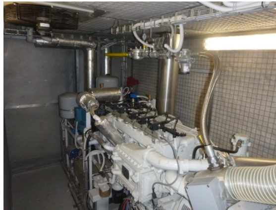
Fig. 5: Combustion engine of the cogeneration unit
