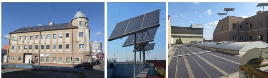
Fig. 2: Three types of photovoltaic panel on the roof of TCO - static panel, tracker and amorphous cells
