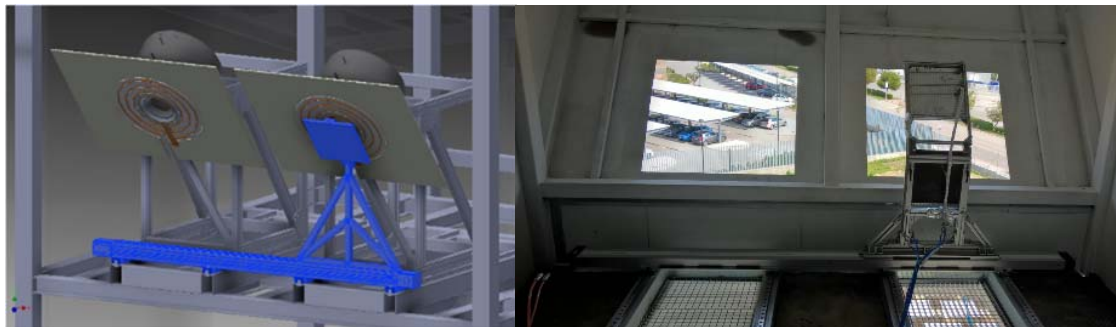
Fig. 5: Left: Technical drawing of the flux measurement system (in blue) in front of one of the receivers. Right: Installation of the flux measurement system at the experimental level of the solar tower (solar reactors not yet installed). The rail at the bottom allows to move the flux measurement system quickly in-between the apertures and into a safe position, the cooling water supply is visible.
