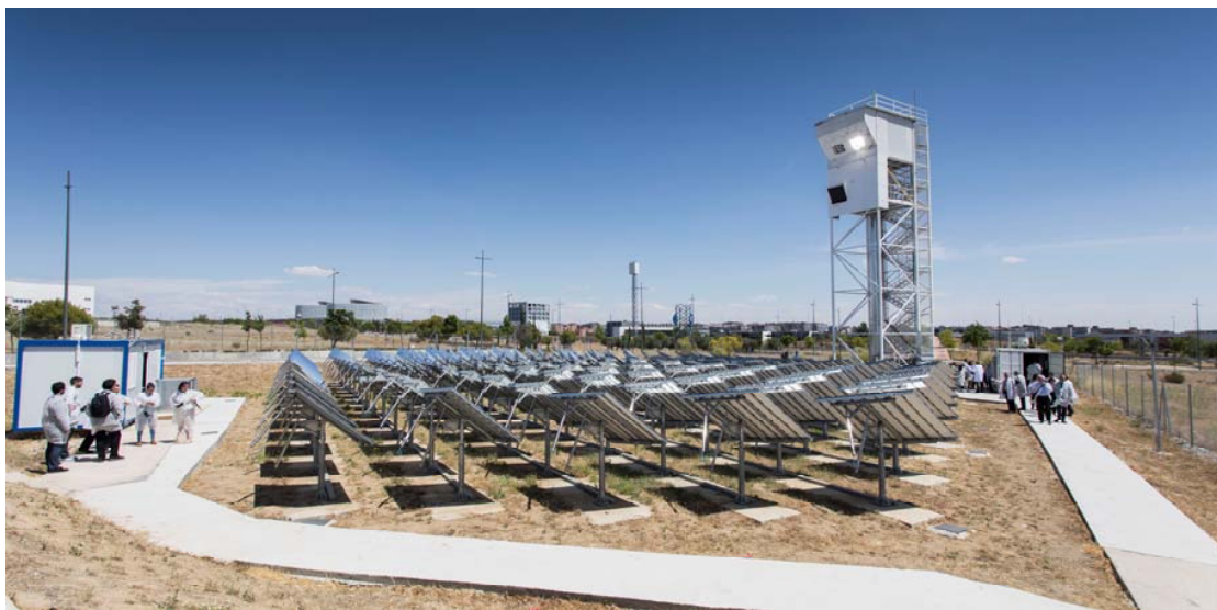
Fig. 11: Heliostat field with 169 heliostats focusing onto solar reactor with ceria located on top of a 15-m tower (optical height). On the right side at ground level the container with the gas-to-liquid conversion plant.
