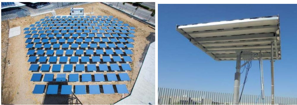
Fig. 4: (Left) Aerial view of the heliostat field from top of the tower. Control room at the rear. (Right) Lateral view of single heliostat of 3m 2 reflecting surface and two rectilinear actuators.
