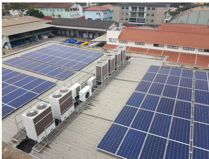
Fig. 7: 36 kWp PV system installed at Sicoob Centro-Serrano headquarters at Santa Maria de Jetibá-ES
