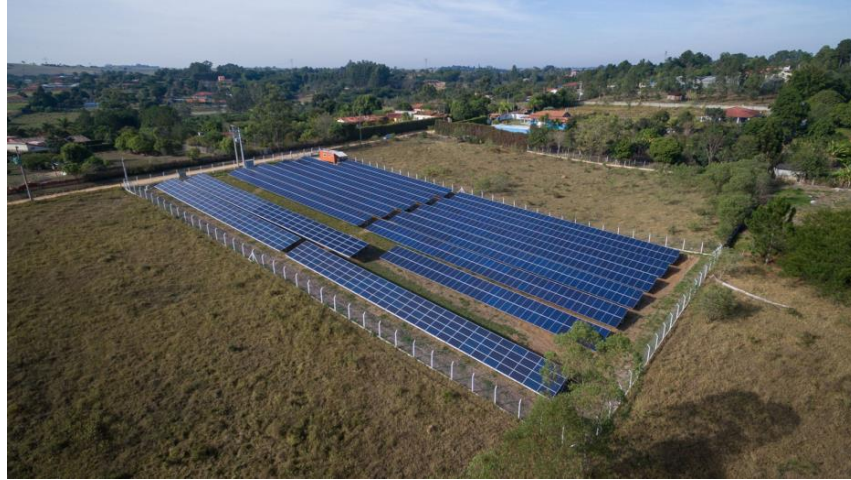
Fig. 5: Compartsol PV power plant, with an installed capacity of 400 kWp
