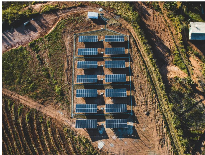
Fig. 4: Enercred power plant currently under construction to be connected to the grid by the end of 2019.
