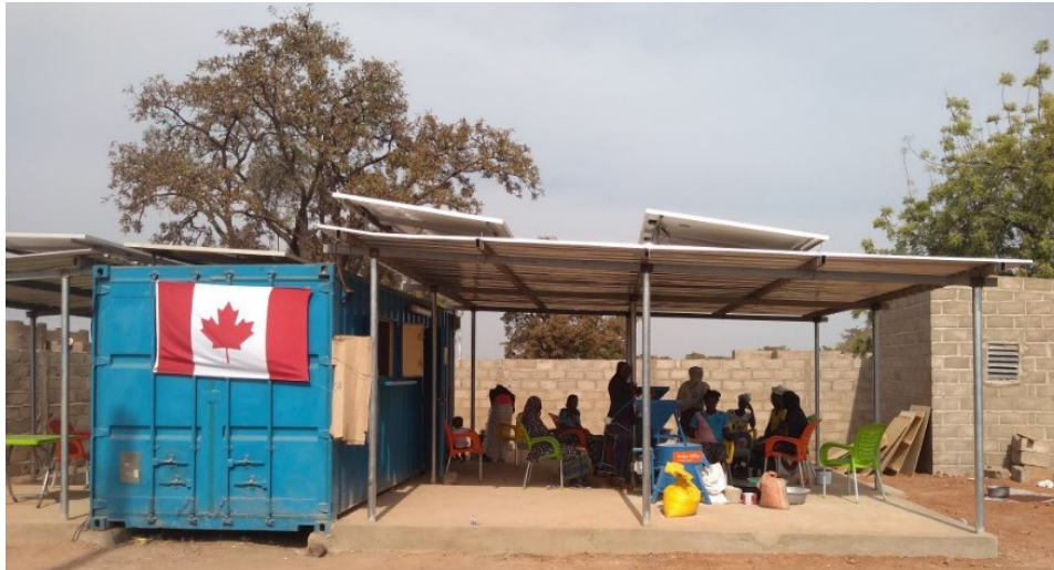
Fig. 2: Photograph of the PV system showing the solar milling equipment on the shaded concrete floor.
