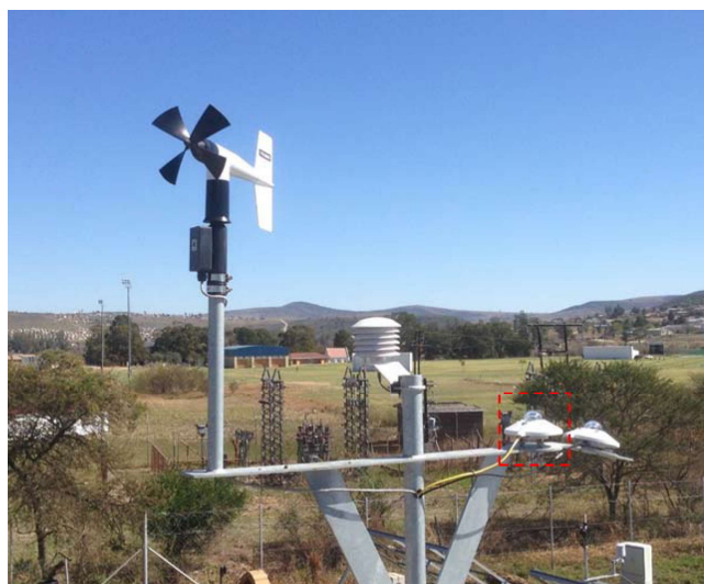
Fig. 2: Setup an outdoor weather station for global horizontal irradiance measurement
