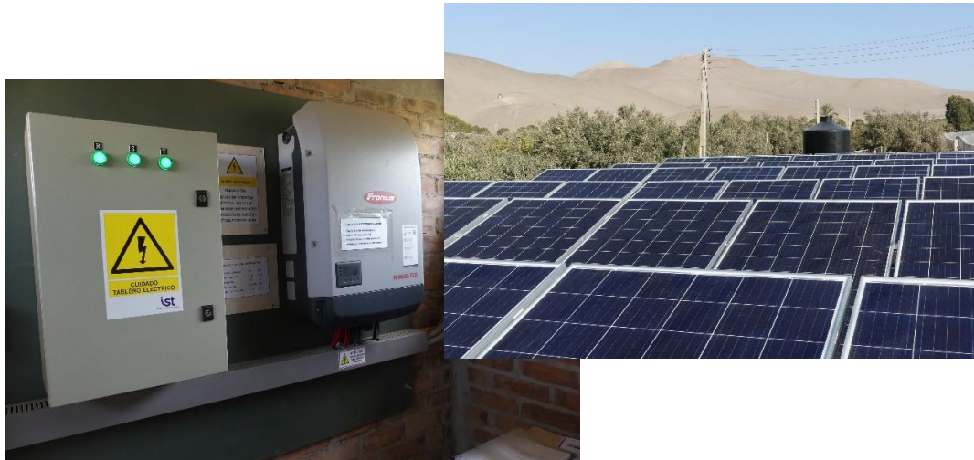
Fig. 5: Principal components of 25 kWp PV on-grid system (Arica, northern Chile)
