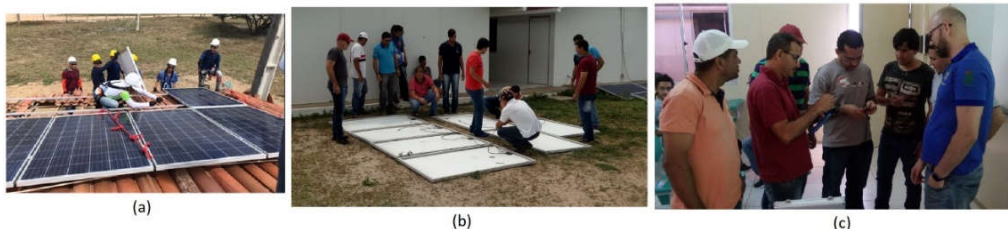
Fig. 3: (a) Modules installation on practice roof, (b) Electrical connection execution based in mechanical layout and (c) MC4 connectors assembly.
