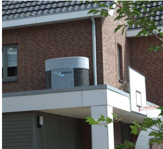
Fig. 9: SolabChiller placed near a family dwelling
