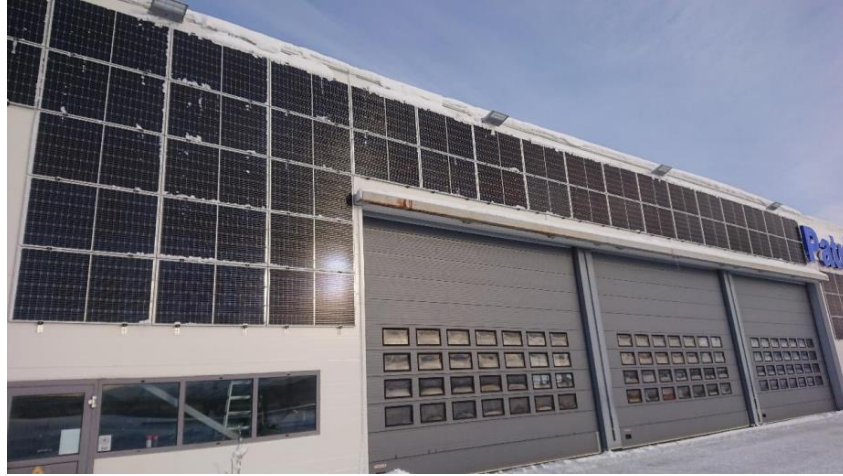
Fig. 2. The 100 m 2 photovoltaic system at Bardufoss Airport. Photo: Clara Good.
