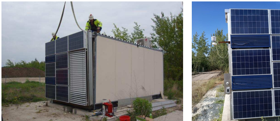
Fig. 3: Installation of autonomous curtain walling façade unit at test cell (CVUT UCEEB)
