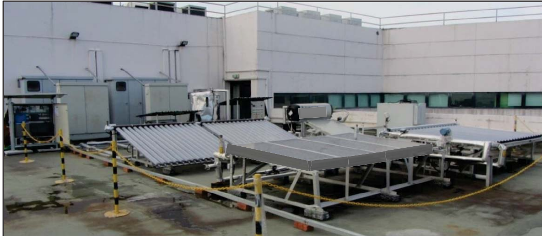
Fig. 1: Solar Thermal collector testing system at the roof top of the Solar Energy Research Institute of Singapore (SERIS). Three different solar thermal collectors were installed for the test operation.
