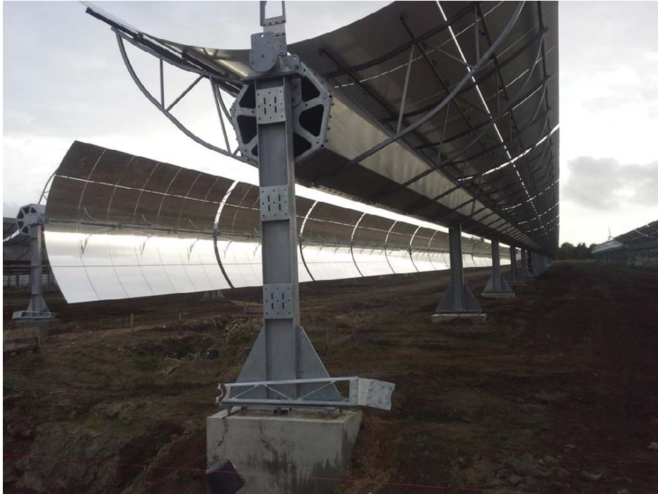
Fig 3. Photo of the CSP collector field, under construction. The collector rows are 240 m long and a total length of 480m of collectors are series connected in each series loop. (No absorbers or connecting pipes are installed in this photo).
