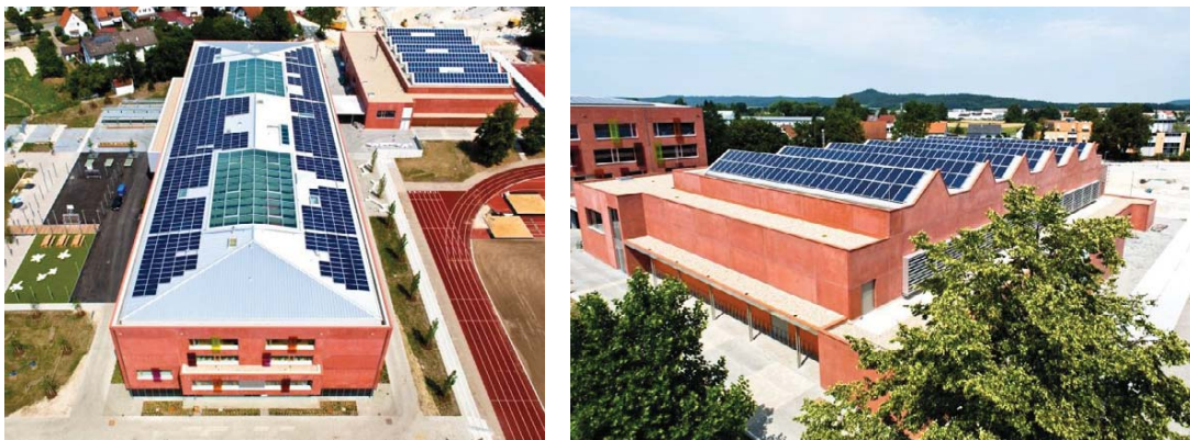
Fig. 5: Aerial photos of the PV-installation on the school building (left) and the gym (right)
