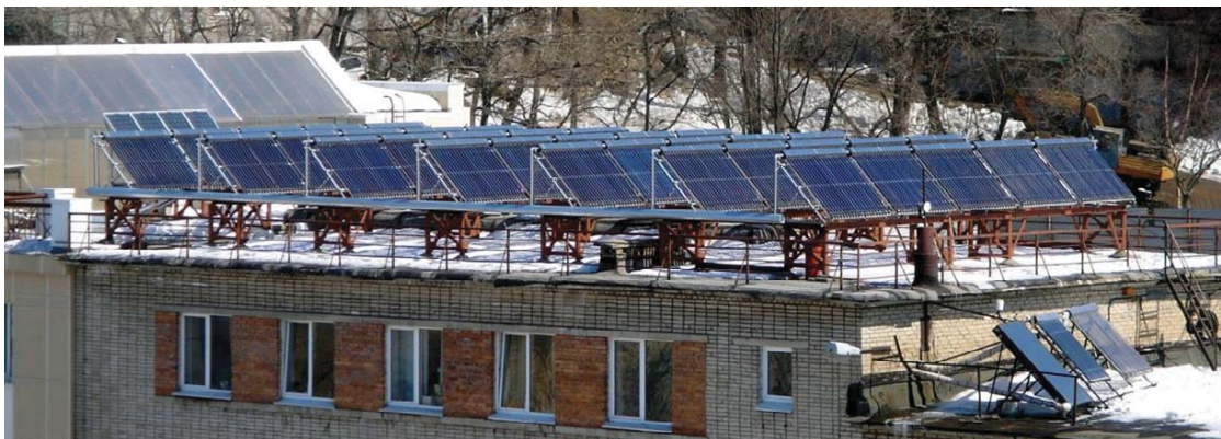
Fig. 12: Experimental solar installation of hot water and heating.
