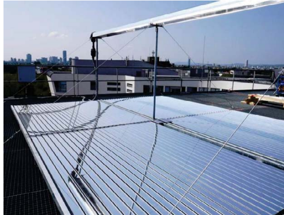
Fig. 4. Installed Fresnel collector [Fresnex, 2015]
