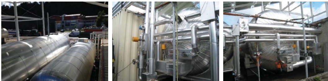
Fig. 2 : Storage tanks of the installation
