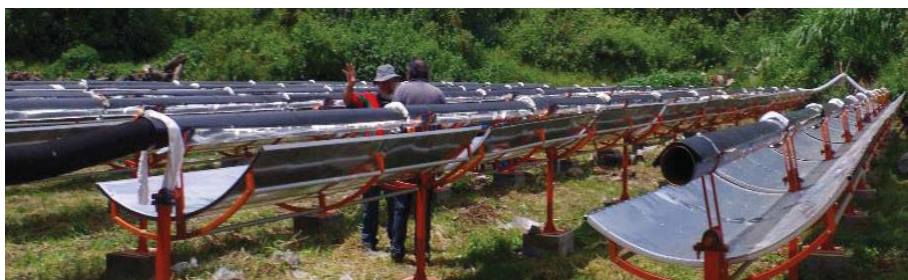
Fig. 1: The solar concentrator's installation in Yanayaco, Cusco, Perú
