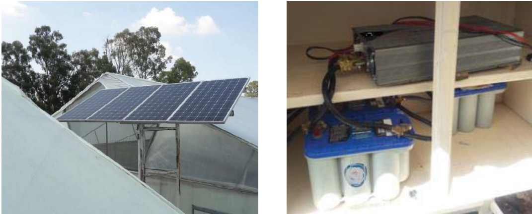
Fig. 3: PV array and hybrid inverter with battery bank.
