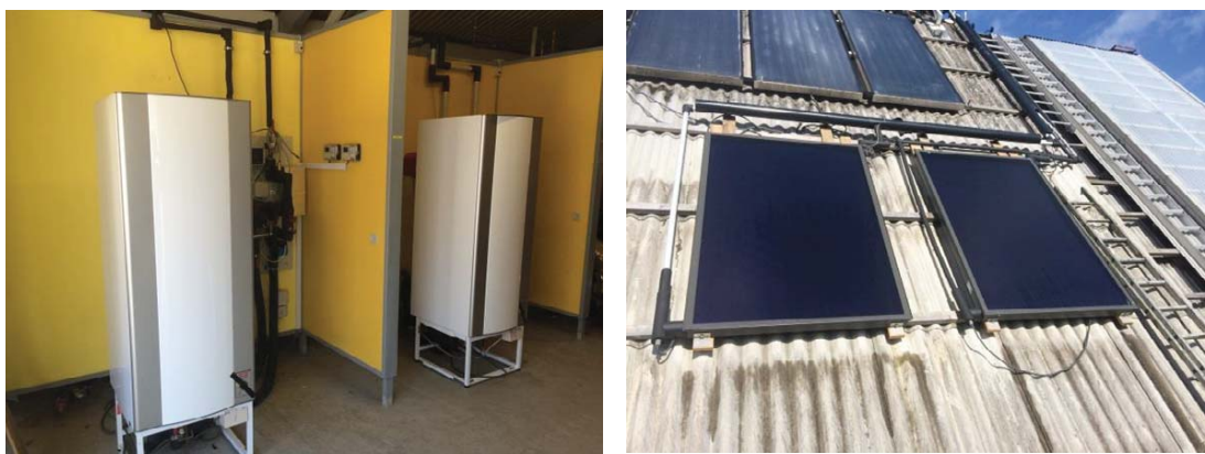
Fig. 2 Pictures of the storage tanks and solar collectors in the two SDHW systems.
