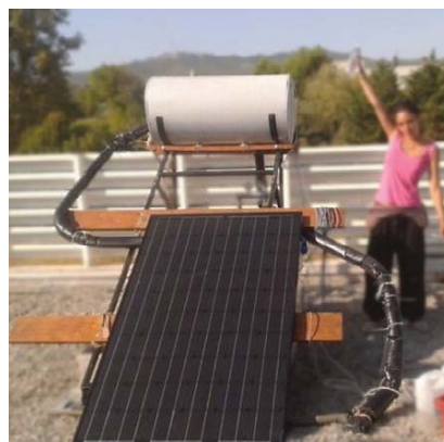
Fig. 1: A DualSun module being installed in a thermosiphon water system testbed in Marseille, France.
