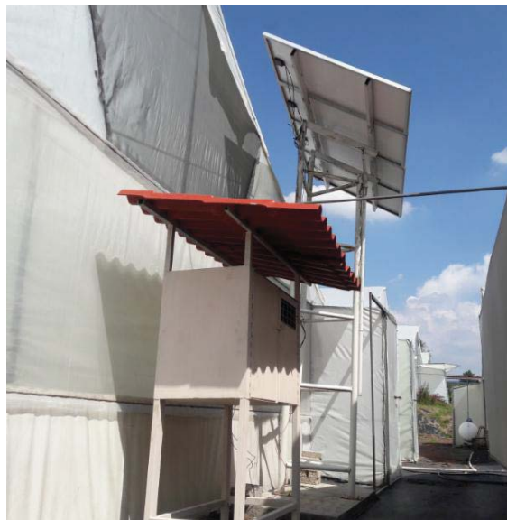
Fig. 4: View of PV system outside greenhouse.
