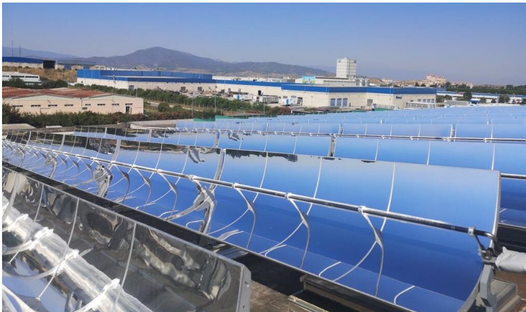
Figure 1 Photo of parabolic trough collectors (Solarthemen Media GmbH, 2021)
