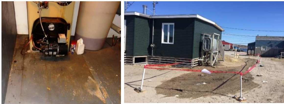
(a) Heating oil leakage from boiler (Photo taken by author)
