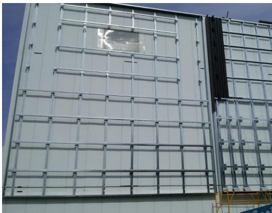
Fig. 3: Transpired solar air collectors under construction at the Canadian National Solar Test Facility.
