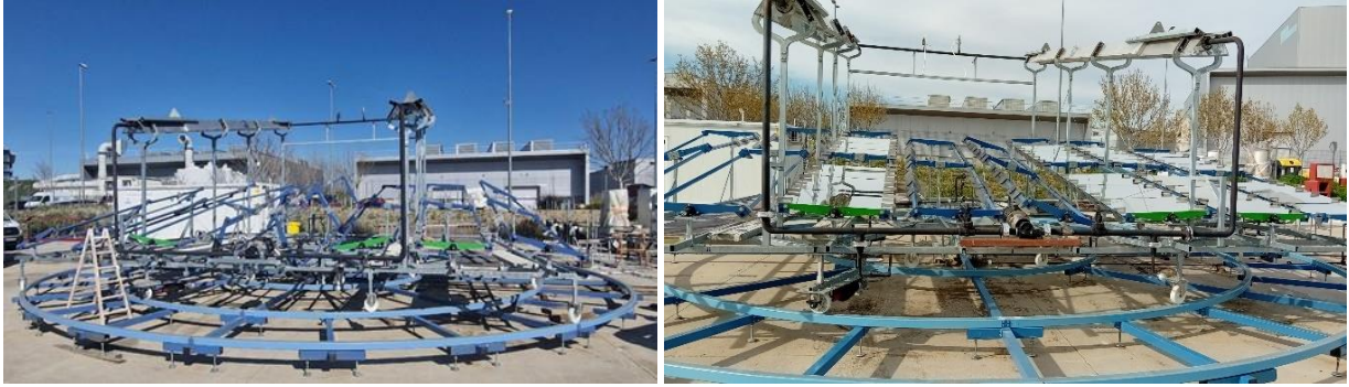
Fig. 7: SunDial with single axis tracking system for the Mandrekas case study, before (left) and after (right) placing the reflectors
