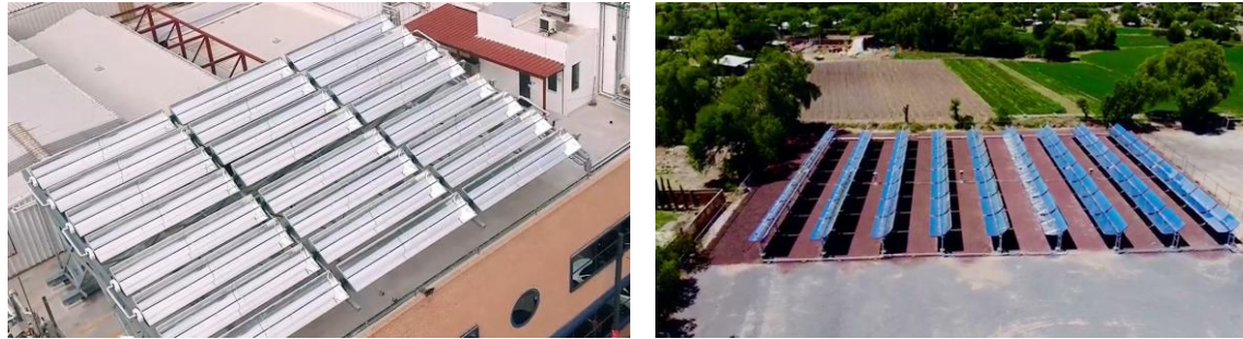
Figure 1212. a) Absolicon's rooftop PTC for IPH application in Greece (RTC, 2023); b) Inventive Power's ground mount application in Mexico (Rosell, 2022). Image Credits: Absolicon and Inventive Power
