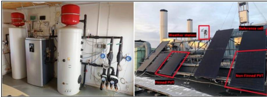
Fig. 1: Left) Mechanical room containing the HP and hot and cold storage tanks, as well as the circulation pumps and their monitoring system. Right) Test rig with the PVT collectors being tested.
