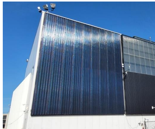
Fig. 4: Installed collectors. left: unglazed, selective surface model, right: two-stage black paint model.
