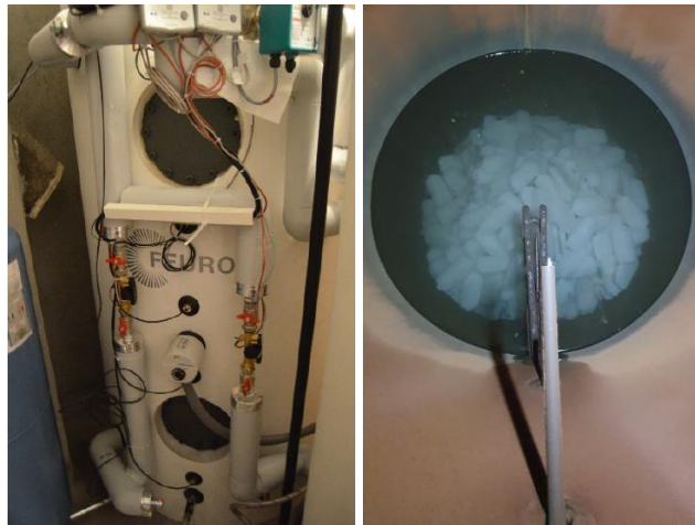
Figure 4: Left 800L buffer boiler. Right: Inside-view of the buffer boiler 30% filled with COWA Capsules.
