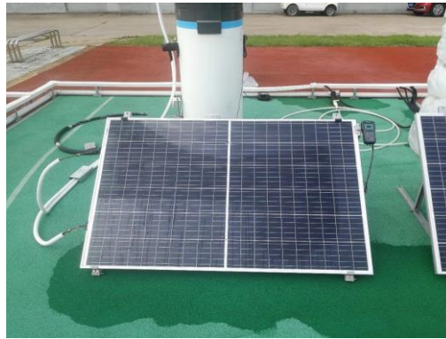
Fig. 8: Prototype of the PVT heat pump water heater system
