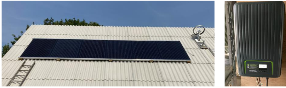
Fig. 3: PV panels on the roof of the test facility (left) and the inverter (right)
