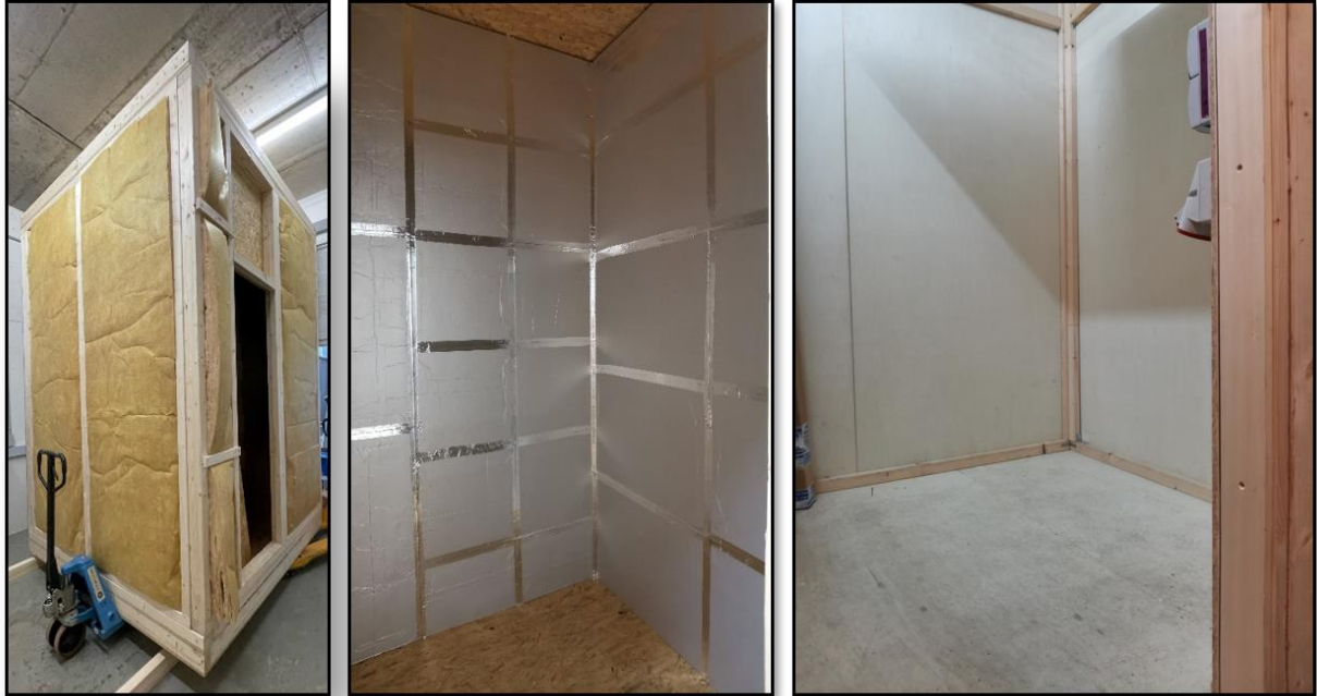
Figure 6: Pictures of the thermally high insulated test chamber. Left: Outside of the chamber with 100 mm mineral wool. Middle: 20 mm vacuum insulation panels installed to the inside of the chamber. Right: Inner top layer of 12 mm multiplex board.
