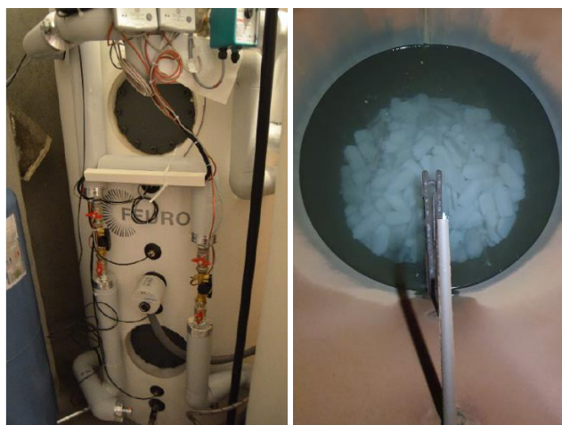
Figure 4: Left: 800L buffer boiler. Right: Inside-view of the buffer boiler 30% filled with COWA Capsules.
