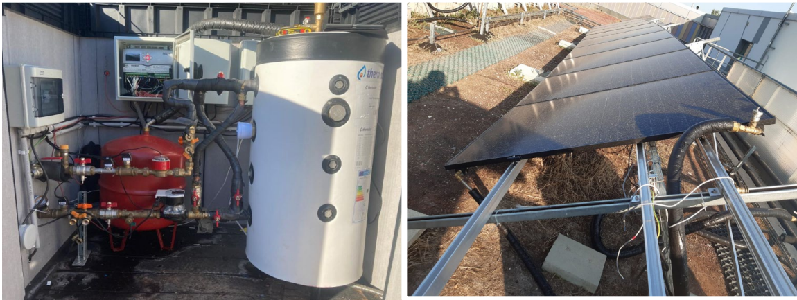
Fig. 2: (a) Photo of the test bench technical room (b) Photo of the row of PVT panels on the flat roof
