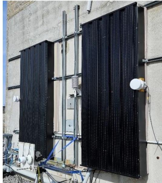
Fig. 3: Collectors mounted vertical on the building's south-facing wall.
