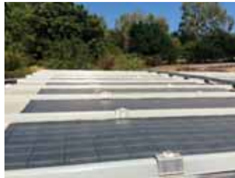
Fig. 7: Naturally washed panels due to rainfall - 3 rd October 2014
