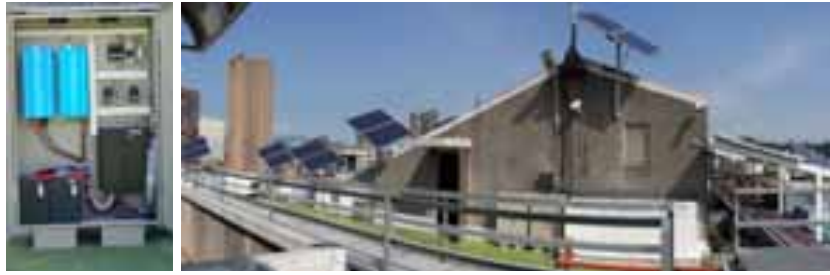
Fig. 3: Hybrid solar PV system for office energy supply.
