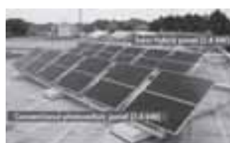
Fig. 3: Appearance of solar hybrid system
