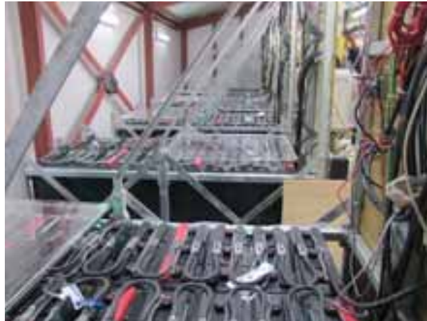
Fig. 3: Crown Battery Banks each at 48 V; 3,747 Ah at a C/20 Discharge Rate
