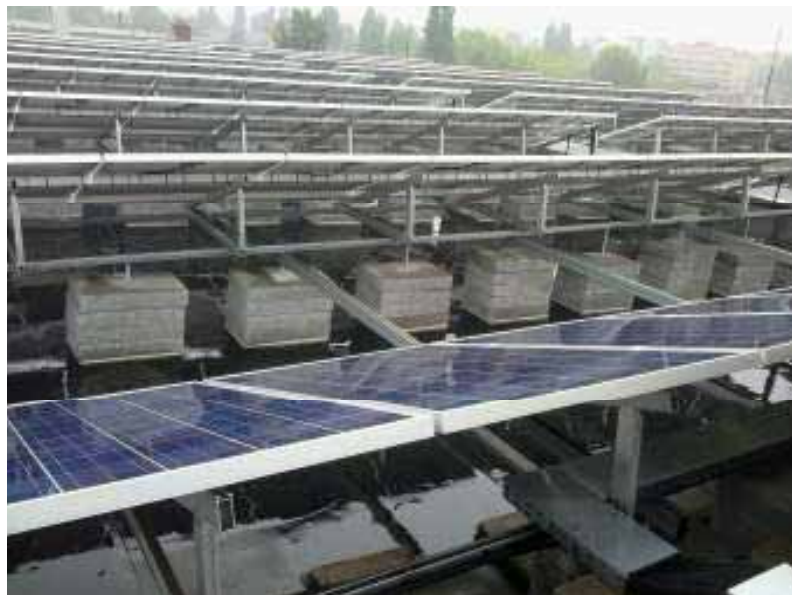
Fig. 2: The examined reference power plant
