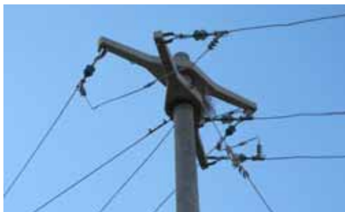
Fig. 4: BREP electrical distribution system as installed by NetCon
