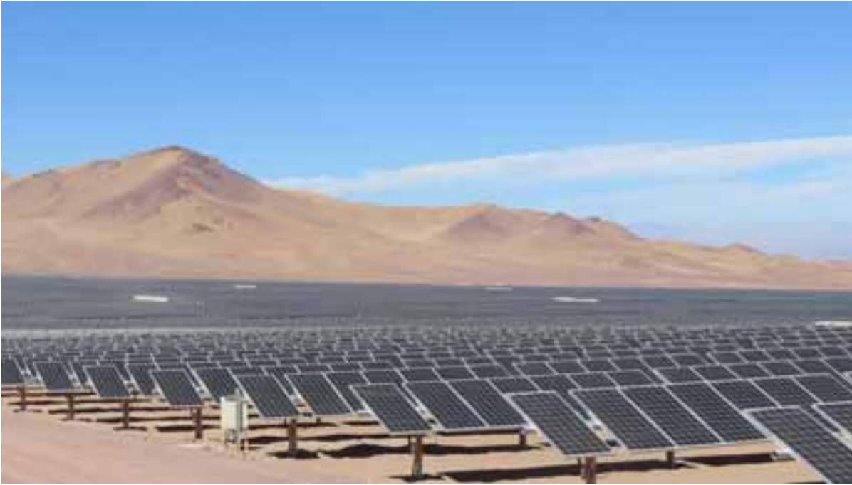
Fig. 4 The “Amanecer Solar” plant. First 100 MW grid tied system in Chile (2014)
