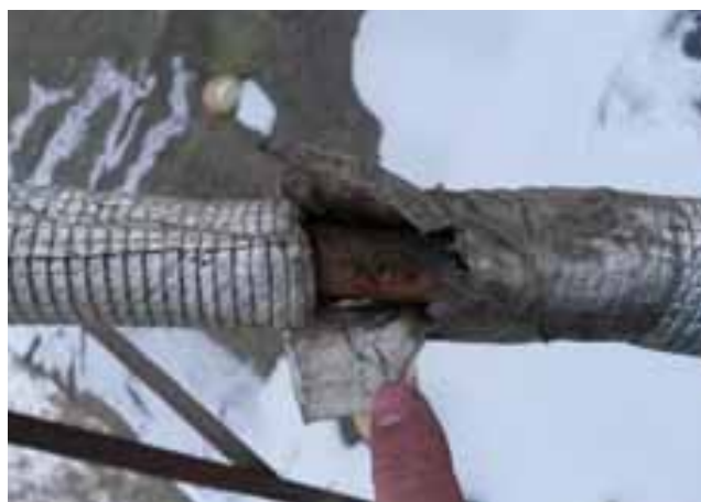
Fig. 8: Three months after heat insulator of solar circuit pipe changed (2014.01.10)
