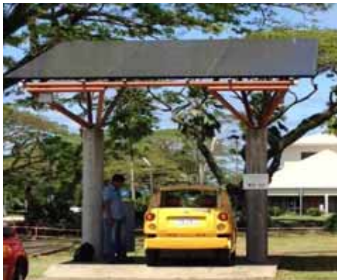
Figure 3.The solar charging station roof mounted panels with two supports to allow for vehicle parking and charging area
