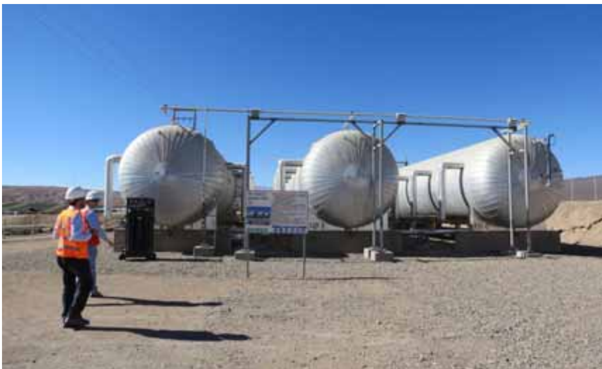
Fig. 6 The “Centinela” parabolic system storage tanks. Each has a capacity of 120 m 3
