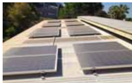
Fig. 2: The installed 5.0 kWp c-Si rooftop system (Auxin AXN-P6T275, Inverter: SunnyBoy SMA SB 5000TL-20)
