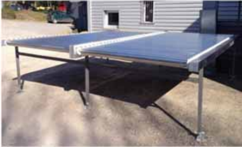
Fig. 8: Pilot ground mounted installation
