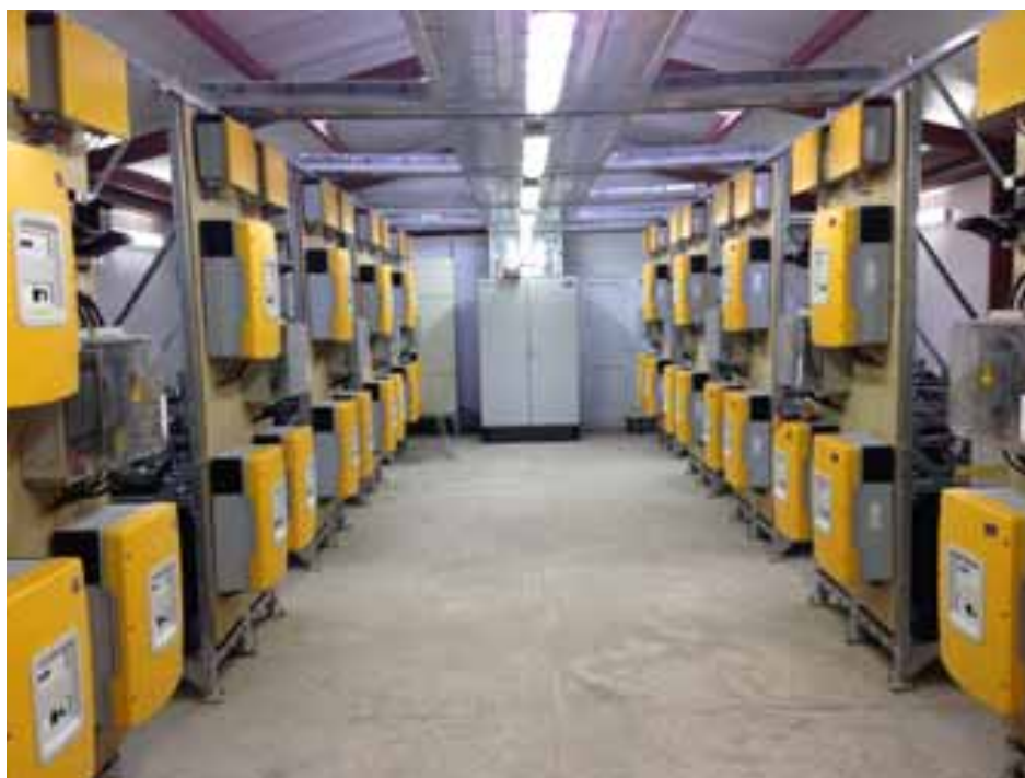
Fig. 5: SMA Multi-cluster Hyderabad BREP Power House with Sunny Island Battery Charging Inverters
