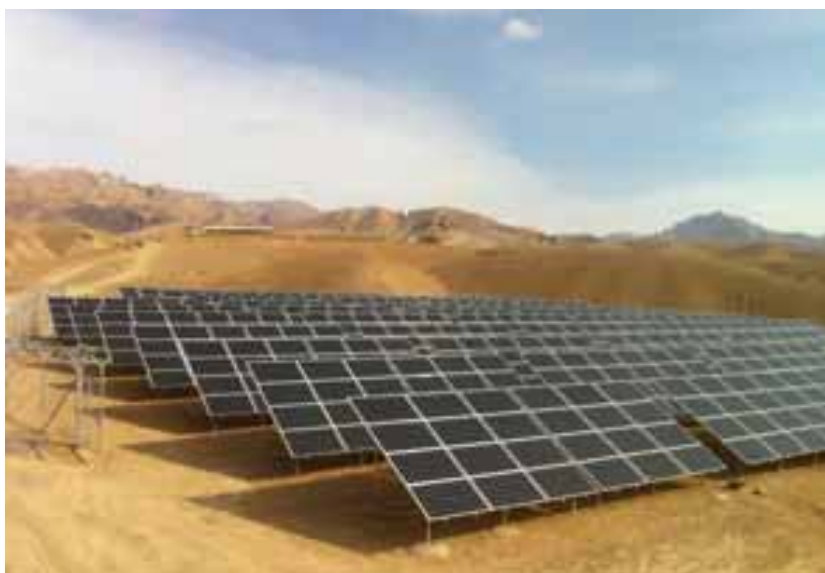
Fig. 2: One of the Large BREP PV Arrays: 300 kWp at the Mullahghulam site
