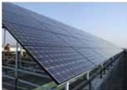
(a) Photo of the installed PV system
