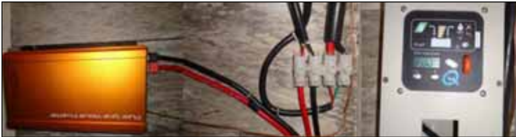
Figure 3: Typical installation of prepaid system and inverter.
