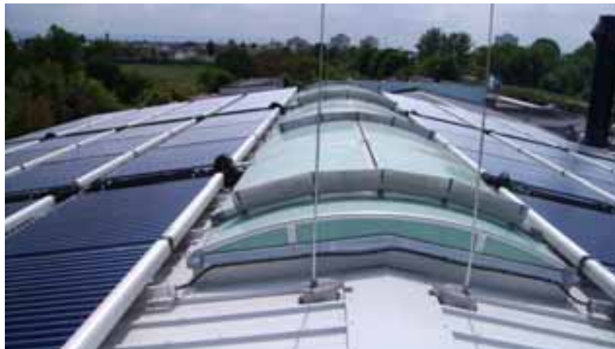
Figure 5: CPC-collector field on metal treatment factory (Holsmölle 2015)
