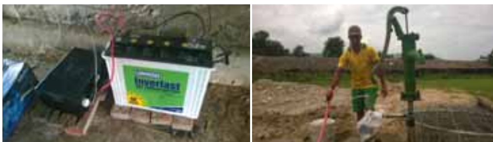
Figs. 15 & 16: PVWP system using a battery and inverter used at a Madi, Chitwan poultry farm in Nepal.
