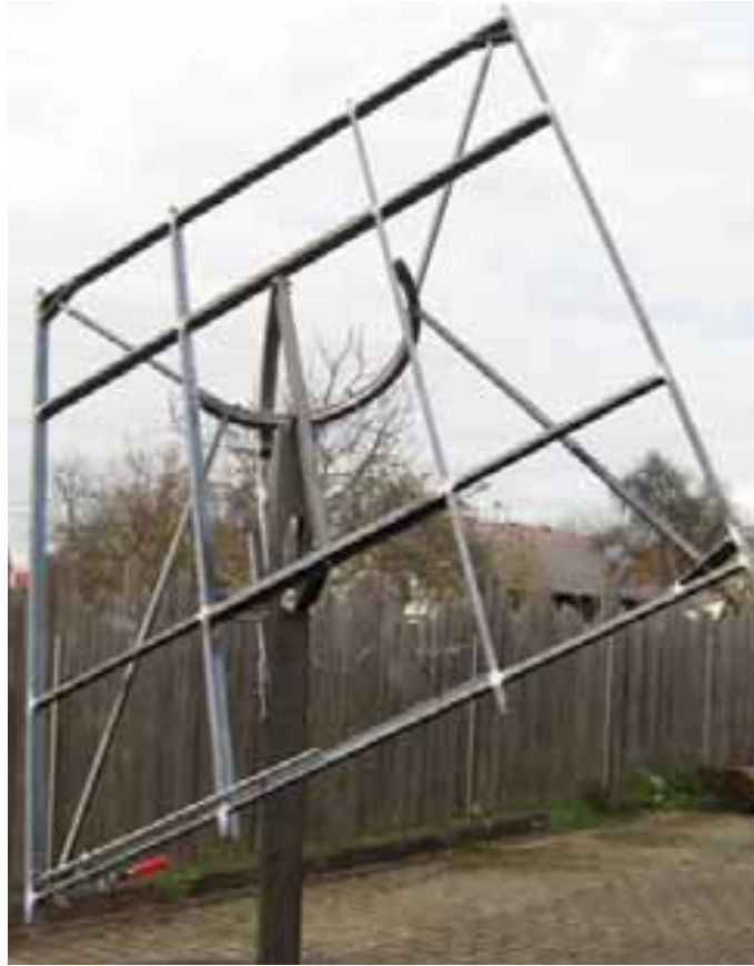
Fig. 10: First frame work mirror support structure with too high flexibility regarding bending about its diagonals.
