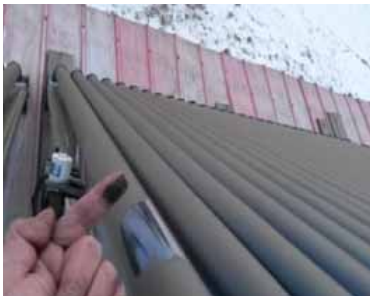
Fig. 7: The glass tube contamination during the measurement (2014.01.10)
