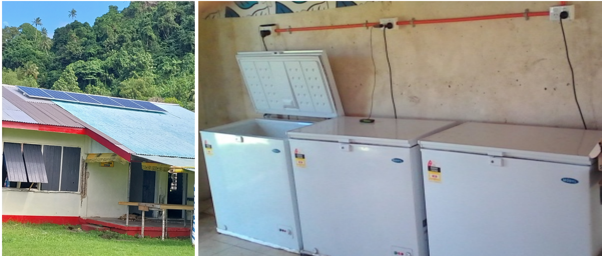
Fig. 4: Solar panels on community hall roof (Left) and freezers (Right)
