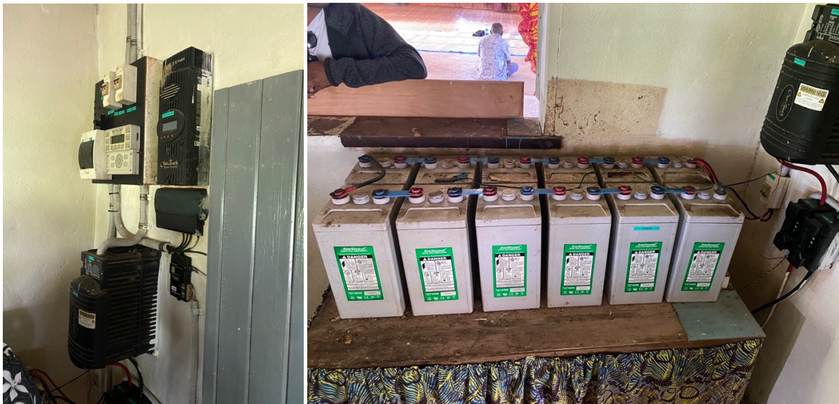
Fig. 5: Electrical components (Left) and uncovered battery bank (Right)
