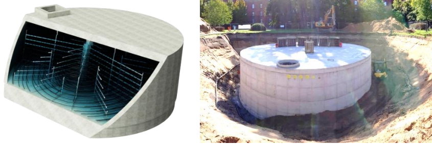
Fig. 1: Concrete tank ice stores. Left: 3D graphic providing an internal view of the ice store, showing the heat exchanger coils and their mounting (LTTT, 2025). Right: photograph taken during the construction phase (Krug, 2019)
