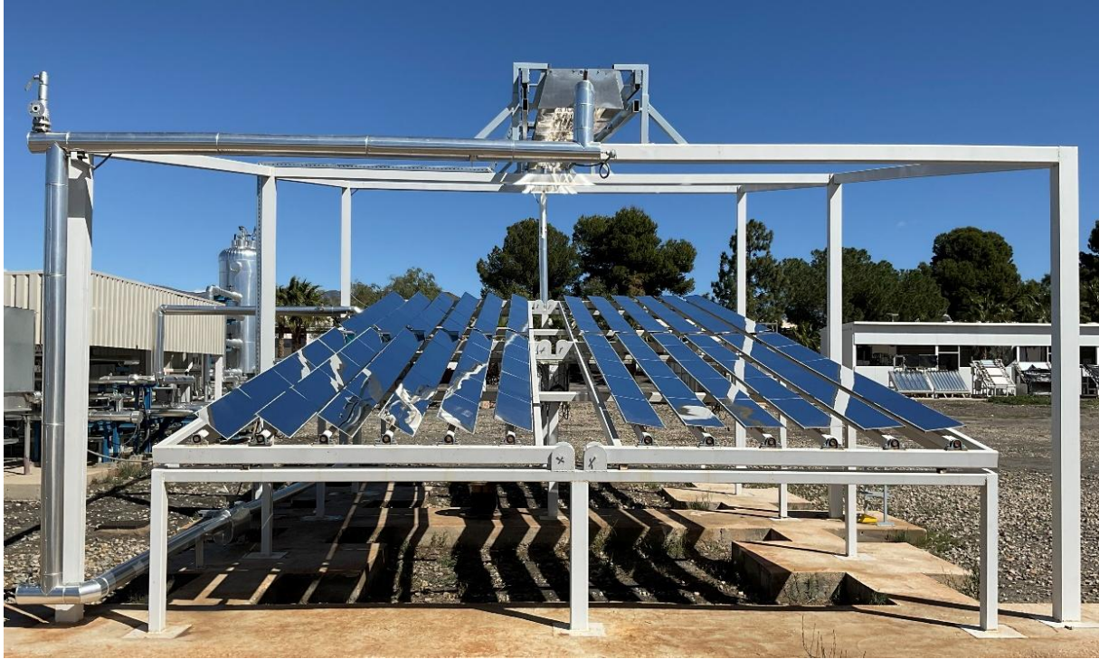
Figure 2: View of the prototype of the innovative linear Fresnel collector installed in Southern Spain.
