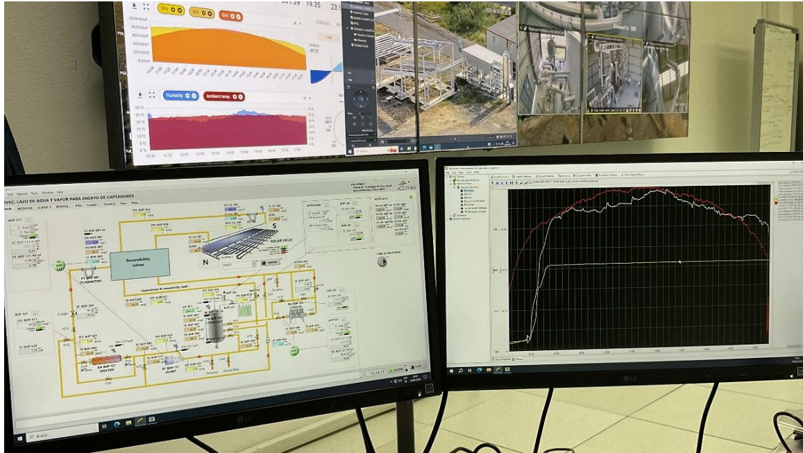
Figure 5: View of the SCADA system of the solar pilot plant during the operation of the LFC prototype on April 24, 2025.
