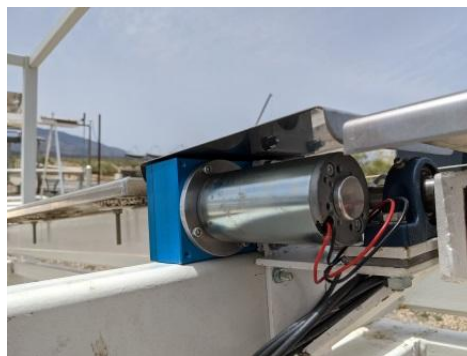
Figure 3: View of one of the gear motors for the drive and control of the LFC facets lines.
