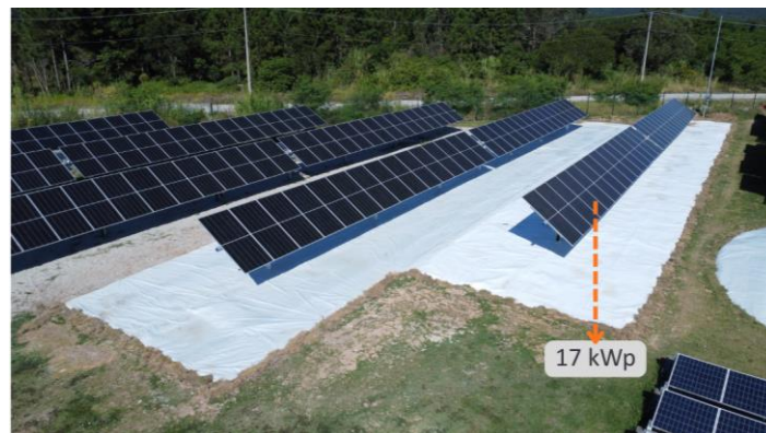
Figure 2: Case study - 17 kWp bifacial solar tracking PV subsystem with white geomembrane ground surface.
