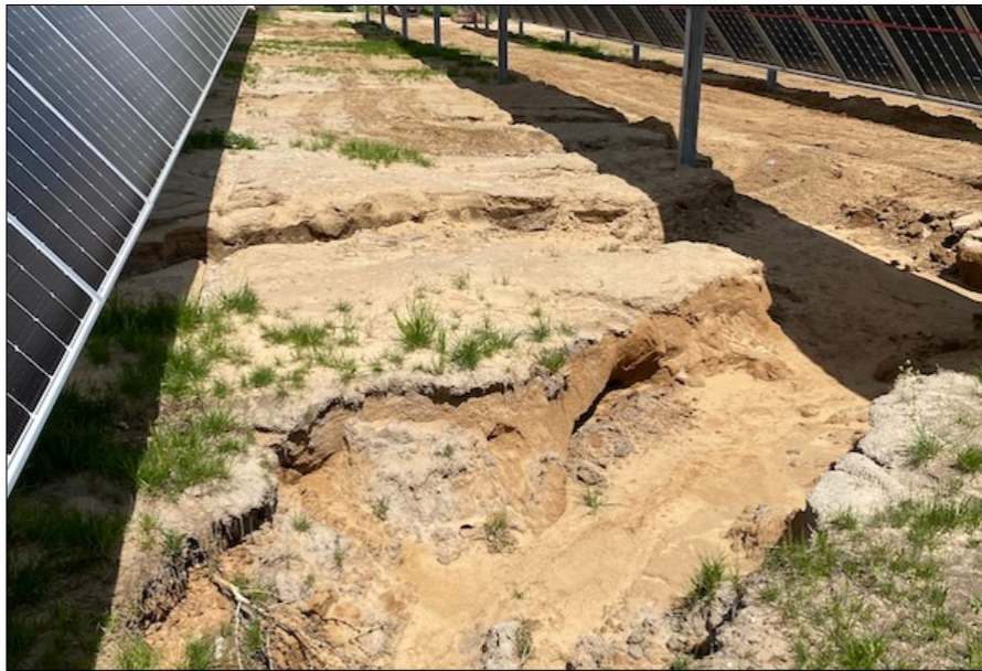
Fig. 2 – Soil instability and erosion (LANCASTER, 2023)
