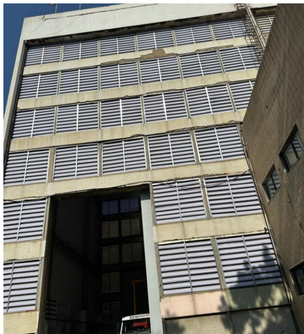
Figure 2: Current state of Block I façade at TC/UFRJ before retrofit.
