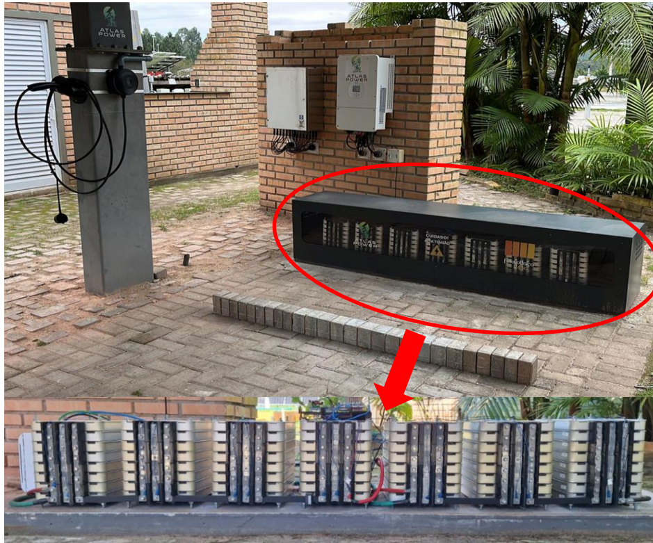
Figure 7. EV charging station equipped with a second-life battery bank composed of 56 repurposed Nissan Leaf modules. The upper panel shows the full installation, including the charger and battery enclosure. The lower panel provides a detailed view of the module arrangement, organized into seven parallel columns, each containing eight modules connected in series.
