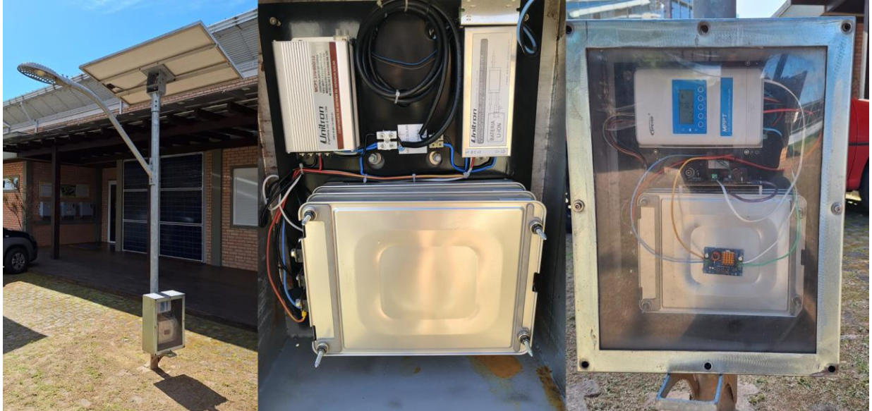
Figure 2. Overview of the solar streetlight test system. (Left) Complete setup currently in operation, including the pole, PV module, and battery enclosure. (Center) First prototype version of the battery compartment and wiring layout. (Right) Updated configuration featuring the MPPT charge controller and improved instrumentation.
