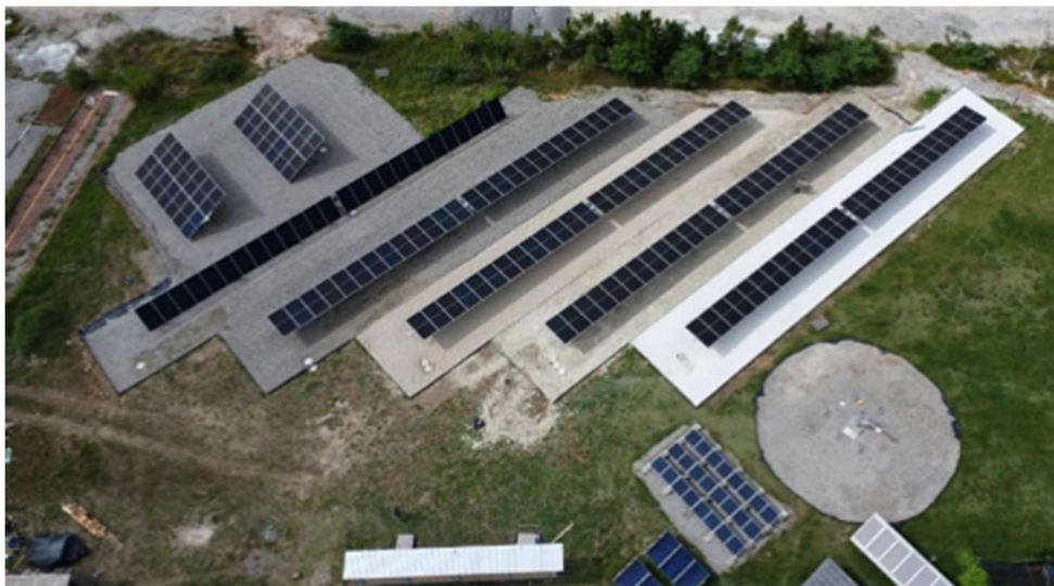
Figure 5: Aerial images of the PV pilot plant used for evaluation of bifacial systems in phase 1.
