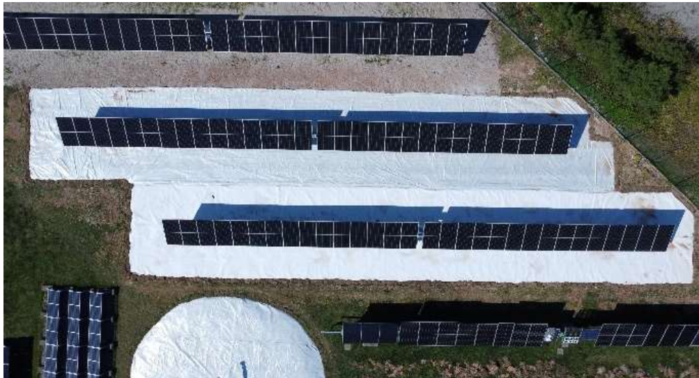
Figure 6: Aerial images of the PV pilot plant used for evaluation of bifacial systems in phase 2.
