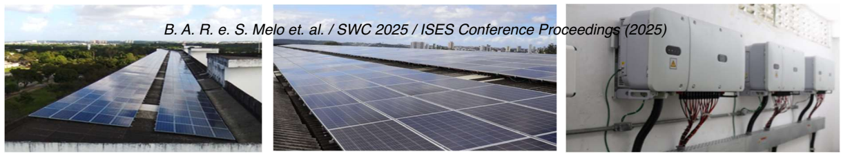
Figure 1: General view of the photovoltaic array composed of 792 p-Si modules (345 Wp each), illustrating partial cloud shading and the group of three 60 kW inverters (Silva et al., 2024).
