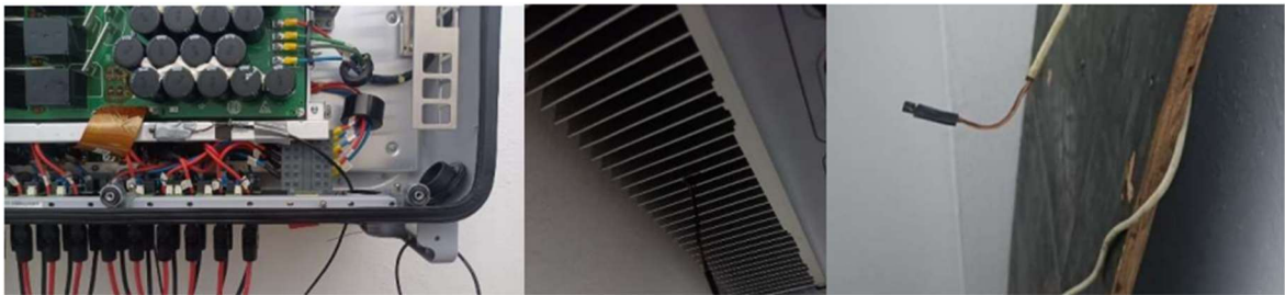
Figure 4: New sensors installation (Silva et al., 2024).
