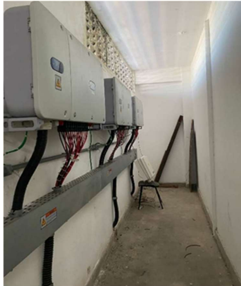
Figure 3: Inverter's installation site in the CTG/UFPE system (Silva et al., 2024).
