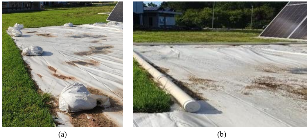
Fig 5: Issues found with the installation methods used for the reflective films: (a) wear and tear of raffia bags and (b) cracks on the PVC pipes. These issues resulted in sand spillage and losses on the films' reflectivity.
