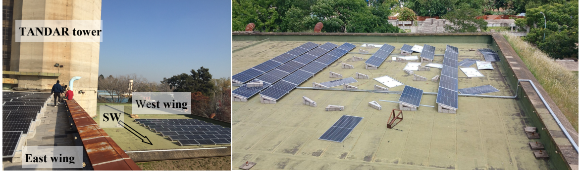
Figure 7: Left: partial view of the 50 kW PV system; on the back of the image, the TANDAR accelerator tower, on the right, the west wing (48 modules). Right: status of the west wing after the storm occurred on 17 December, 2023. South-West direction is indicated.
