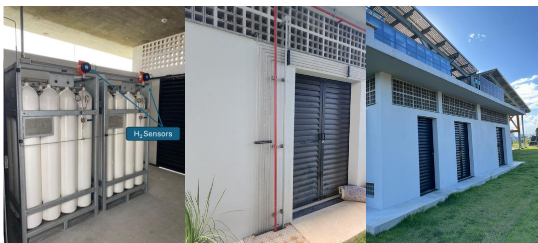
Figure 7: External storage gas housing for hydrogen (left image) and other gases.
