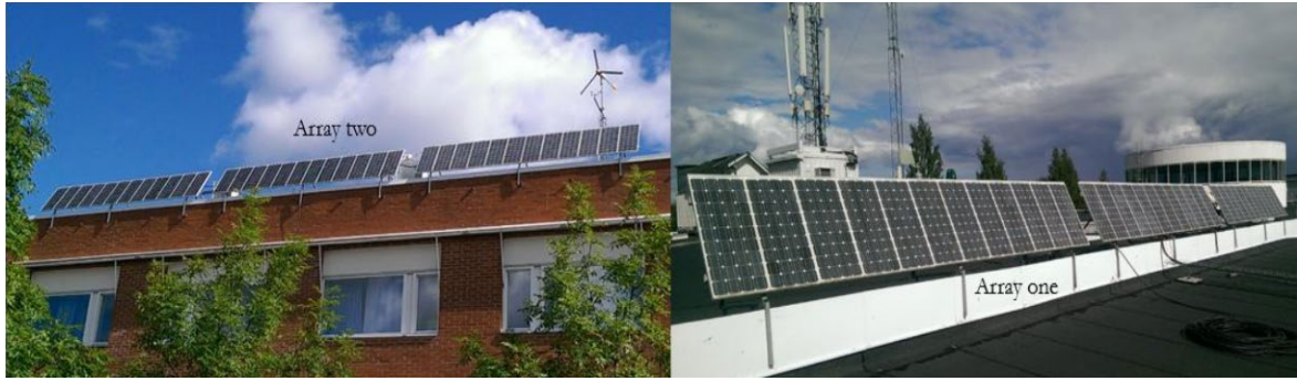
Fig. 1: The BAPV system installed on a rooftop in Sweden in 1994.
