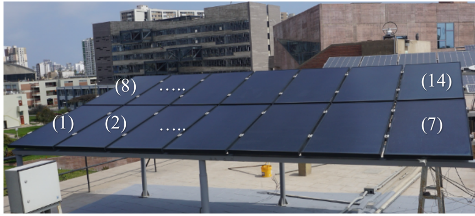
Fig. 1: CIGS system installed in Lima, numbered for EL and I-V curve analysis; identical systems are installed at all locations.
