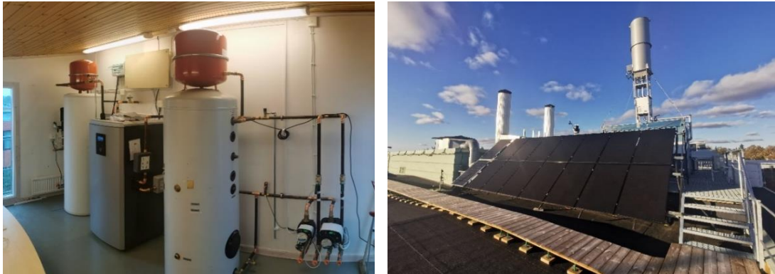
Fig. 1. Testing facility with mechanical room (left) and PVT collectors (right)
